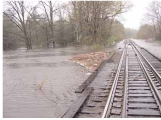
Trestle under water level after May rainstorms
