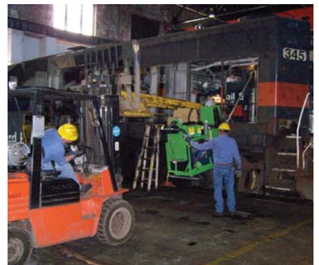
Sheetmetal worker Harvey Johnston (left) and Boilermaker Wayne Plummer (right) prepare to install an APU into locomotive 345. Photo by Mike Slaney
