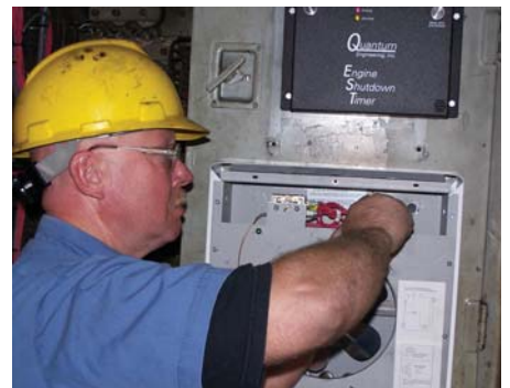
Electrician Cameron Gallo installs an auxiliary electric cab heater in the cab of locomotive 345. Note the Engine Shutdown Timer (EST) at top of photo. Photo by Mike Slaney
