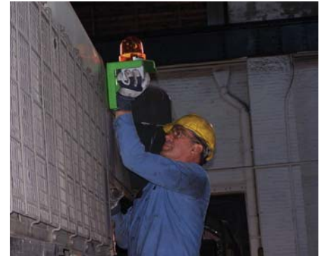
Boilermaker Wayne Plummer installs the APU fault alarm beacon near the roof line of locomotive 345. Photo by Mike Slaney
